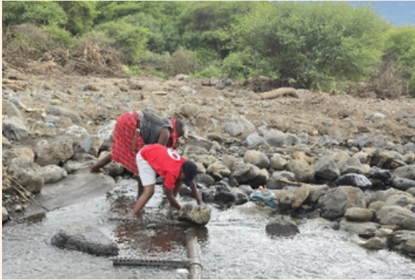
Temporary pipeline to community tank
